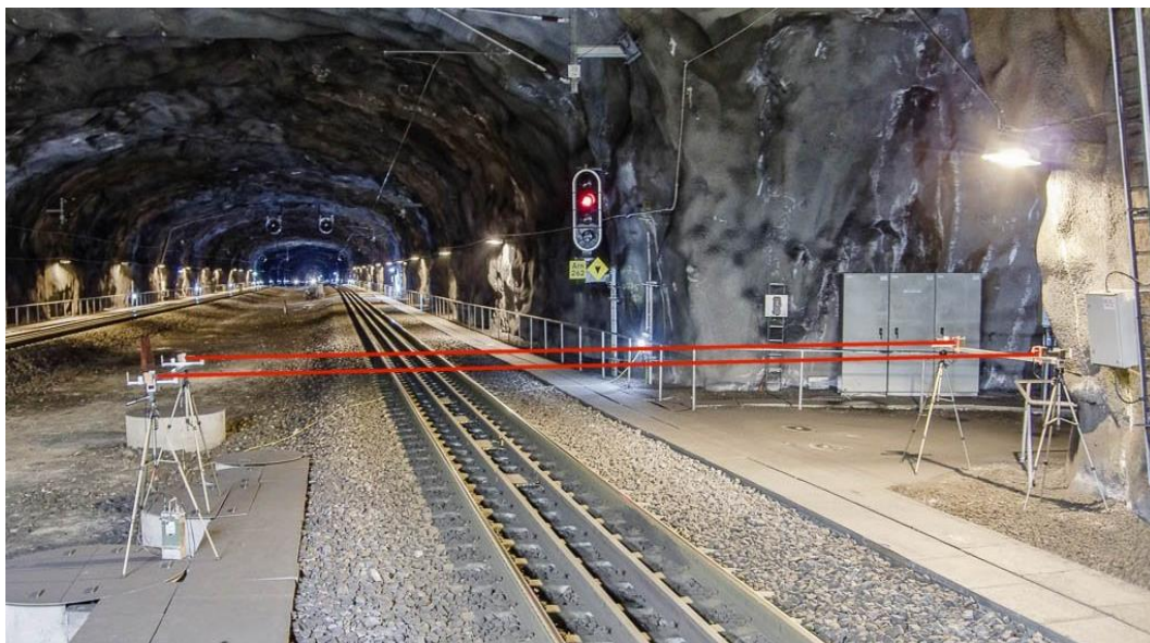
Figure 1: Train traffic counting equipment in the tunnel. Measurement rays across the rail is indicated by red lines in the photo.
