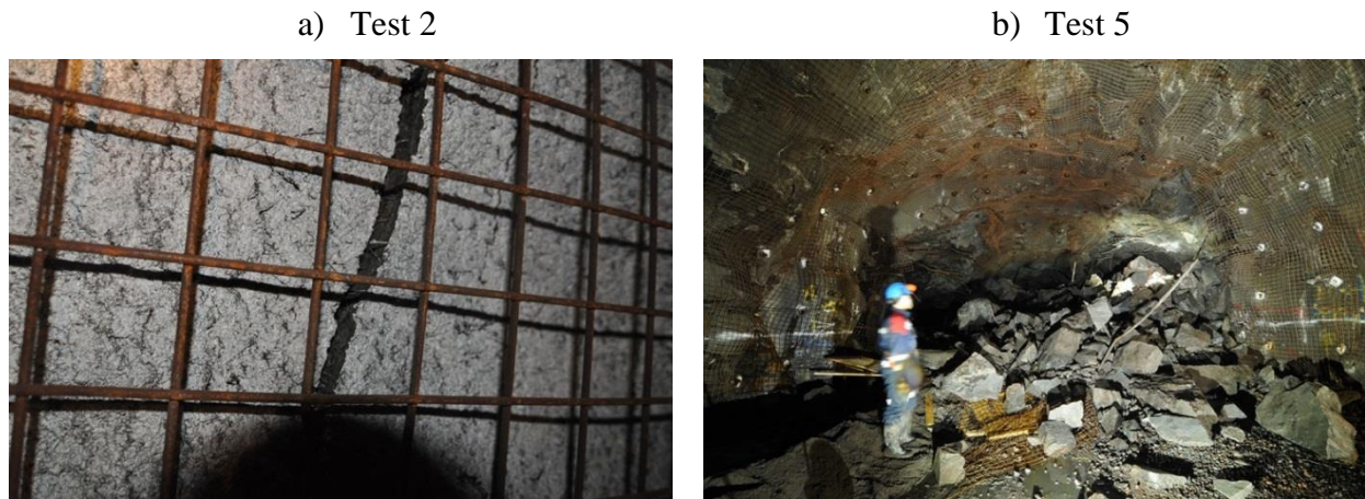
Figure 3: (a) Developed crack on the surface of shotcrete in Test 2 (b) destroyed burden in Test 5 (Shirzadegan et al. 2016a)
