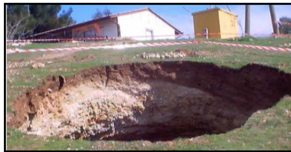
Fig.9: Left photo show the Ground settlement before the full development of the left bank sinkhole.
