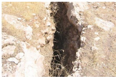
Fig.11: Upstream right abutment, open fissure resulting from slab sliding.
