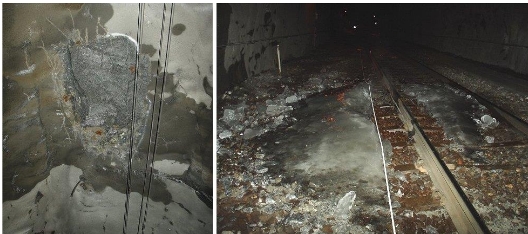
Figure 20: Exposed rock surface after scrapping of shotcrete and ice layer at the track, Glödborget tunnel chainage km 816+597, 2005-01-20
