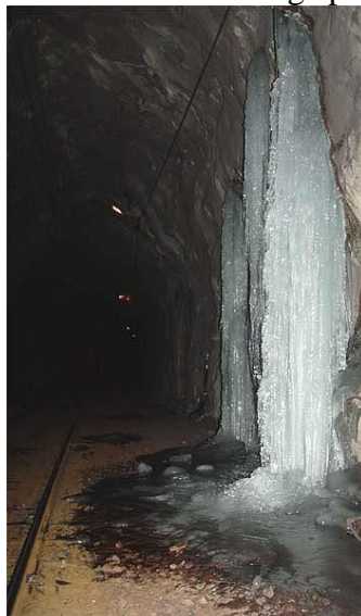
Figure 10: Ice pillar, Nuolja chainage km 1512+284 right, 2004-12-07
