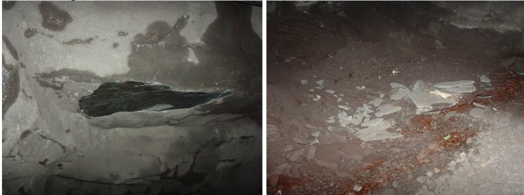
Figure 11: Fall out of shotcrete in roof, Nuolja chainage km 1512+210 roof on the left side, 2004-10-06
