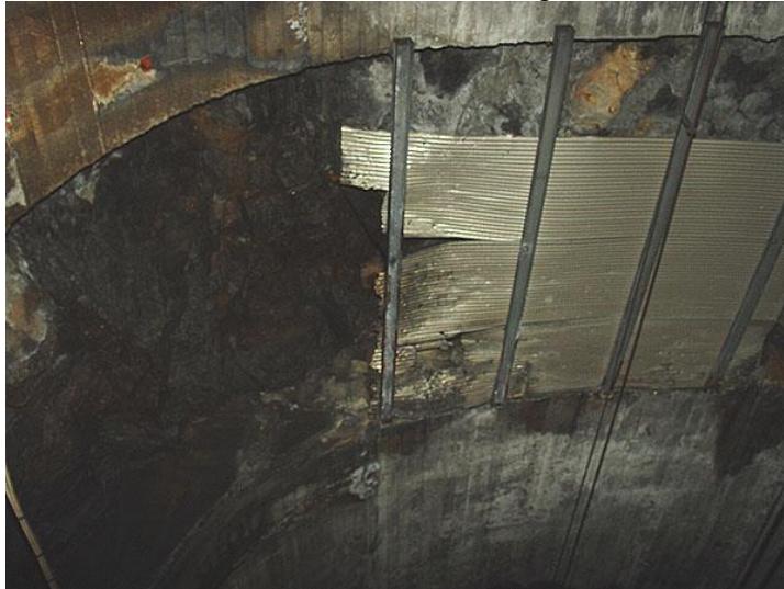
Figure 26: Sheet metal lying on beams between the concrete arches, Rönninge South chainage km 29+730, 2004-12-16
