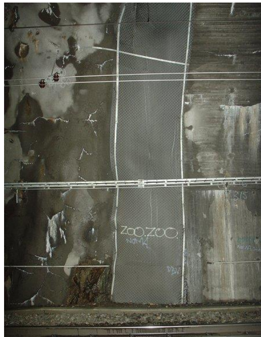
Figure 32: Uncovered drain, Kvedesta North chainage km 39+241 right, 2004-12-17
