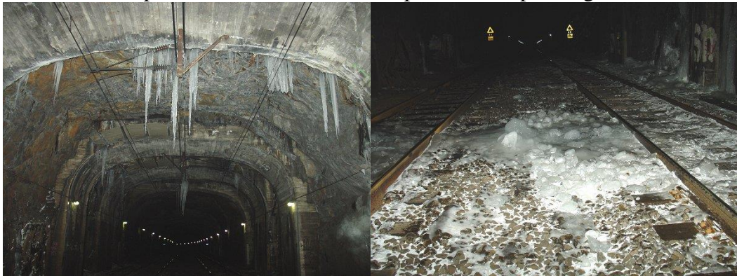
Figure 28: Icicles at an active leakage point and ice layers on the tracks, Rönninge South chainage km 29+720 the first picture photographed to the south, the second to the north, 2005-02-25
