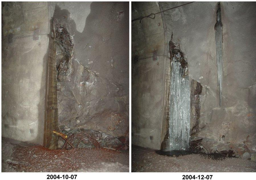
Figure 13: Water leakage where the rock and the concrete arches are connected. Nuolja chainage km 1512 + 626
