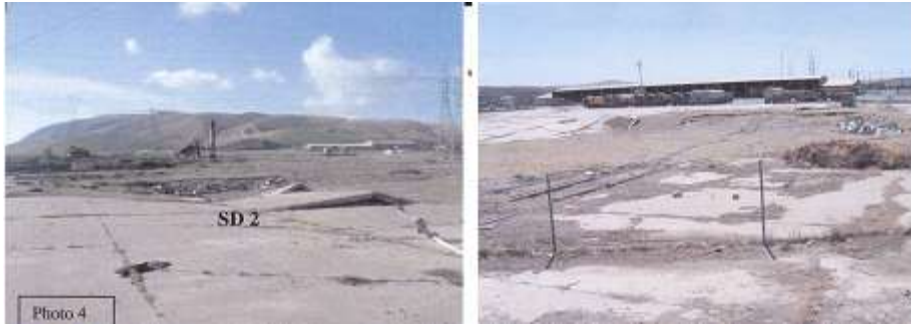
Figure 21: shows Sinkhole SD2 in the contractor paved yard before cleaning and after cleaning of these sinkholes.
