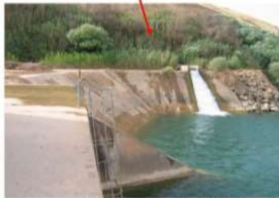
Close-up view of seepage at the Mosul Dam
