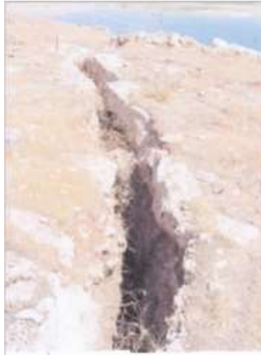
Figure 19: Open fissure indicating slide slab movement at close proximity to right abutment resulting from underground dissolution.
