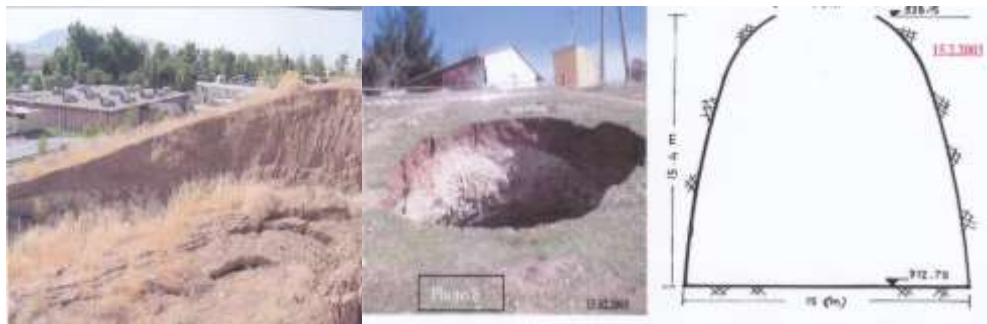
Figure 24: Left: Sinkhole before removing the collapsed material .Middle: After Cleaning: Right: sinkhole sketch showing dimensions.
