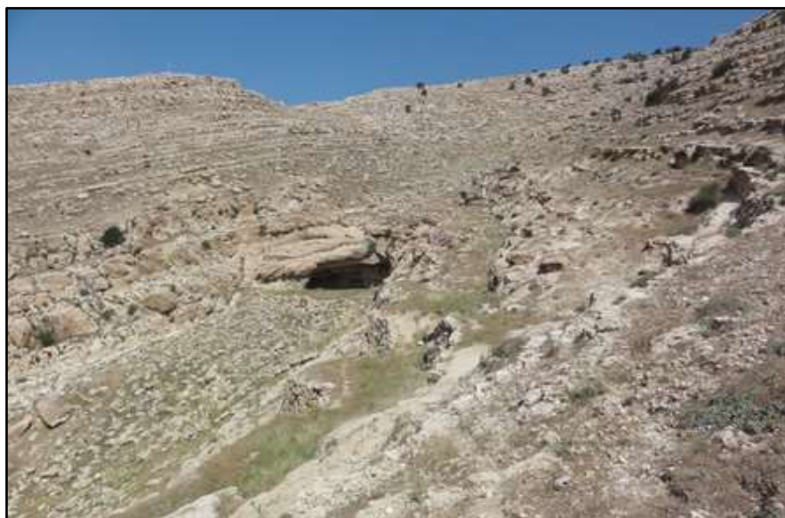
Fig.6: Note the smashed surface of the shear plane of the main slide
