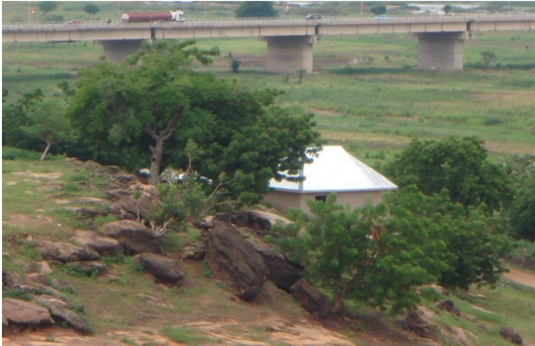
Photograph 2: Boulders sliding down slope due to soil creep placing the building shown at risk. At background is Jimeta bridge over the Benue, the bridge spans 1.4 km.
