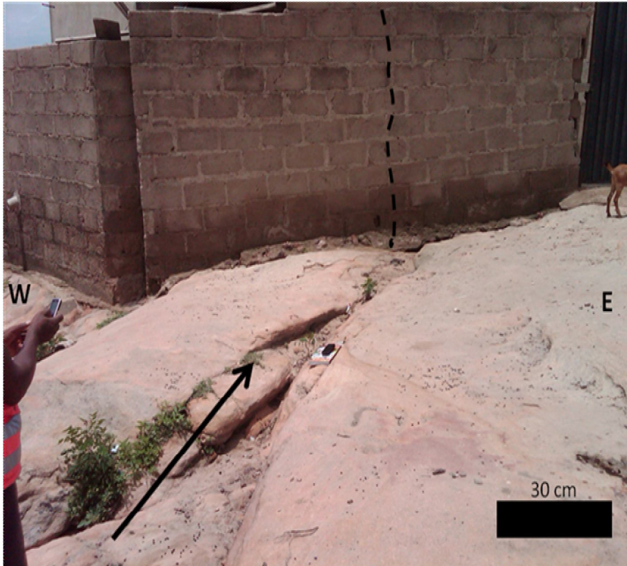
Photograph 5: Wall of building constructed over a fault zone. The wall has cracked at position indicated by broken line over fault trend. Fault trend is N50°E.
