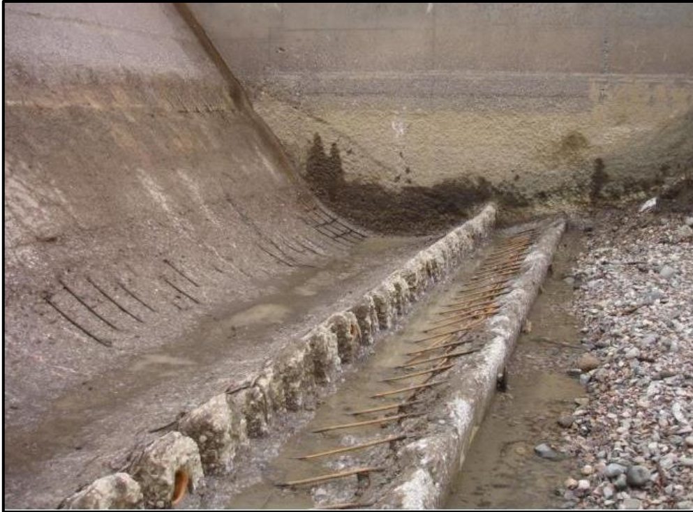
Figure 14: Abrasion erosion damage to the flip bucket and energy dissipaters.
