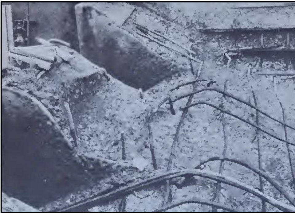
Figure 11: Abrasion erosion on concrete in the dentates, walls, and floors of the Yellowtail Afterbay Dam Sluiceway stilling basin. The “ball mill” action of cobbles, gravels, and sand in turbulent water abraded the concrete, thus destroying the integrity of the structure.
