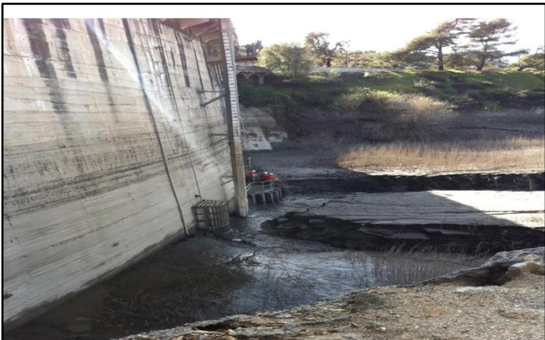
Figure 4: Sediments Threatening Sluice Gate Post- Station Fires of 2009 (Photograph dated on 3rd October 2010) [6].
