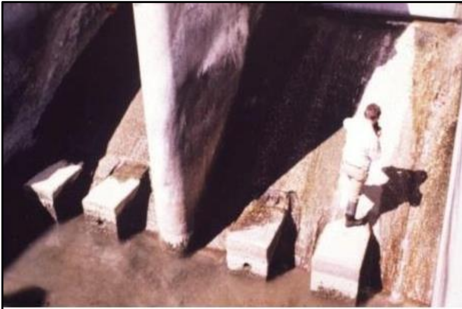
Figure 12: Sand has abraded the spillway at the Milburn Diversion Dam near Sargent, Nebraska [18].
