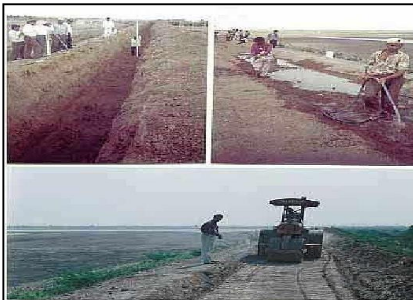
Figure 7: Treatment of longitudinal deep crack at Dam Crest [50].
